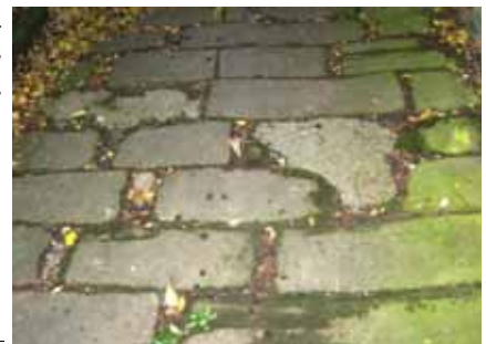
Surviving stone flagged and setted surfaces are at risk from patch repairs in tarmac
