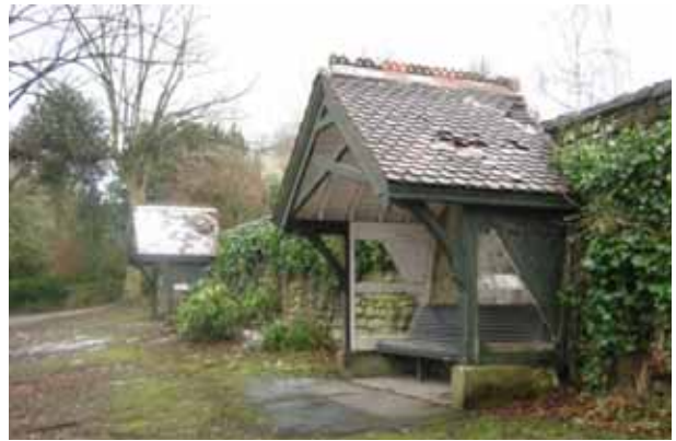
Sadly the covered seating areas in the gardens at County Hall are one of the few surviving remnants of Smedley's hydro grounds, and are deteriorating rapidly
