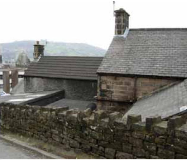
The contrast between roof materials can be seen clearly here. The older Welsh slate roofs with a natural variation in colour are on the right and the later concrete tiles on the left are larger and thicker and more regular in colour and profile
