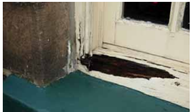
This timber cill has been allowed to rot to the point where a substantial amount would need to be replaced to obtain a good repair. Original joinery is well worth maintaining as it is likely to be of a higher quality than the timber available for windows today
